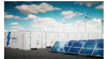
Energy Storage System
