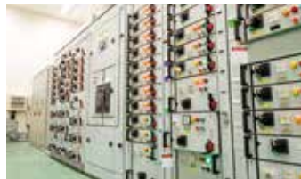
Power Distribution Control
