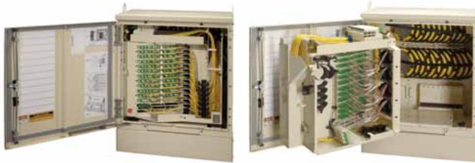
Ground Mount Small 288 Configuration with In-Hub Distribution Cable Splicing
