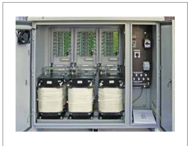
Internal view of an Outdoor Isolating AVR
