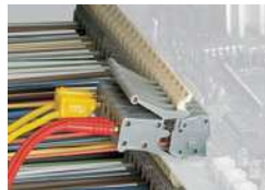
Testing with test plug modules.
