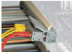
Testing with test plug modules.
