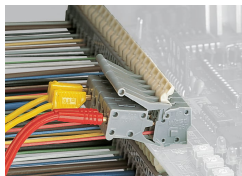
Testing with test plug modules.
