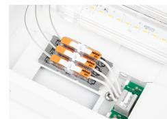
Multi-pole, fixed lighting fixture wiring
