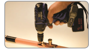
Copper Shear bolt connector installed on EPR insulated 4/0 kcmil 15 kV cable
